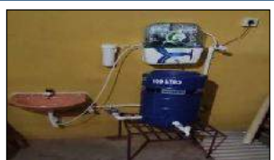
DRINKING WATER SYSTEM
