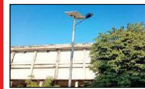
SOLAR STREET LIGHT
