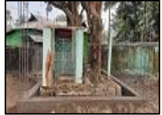
PUBLIC UTILITY AREA AT GOURI KOUN
